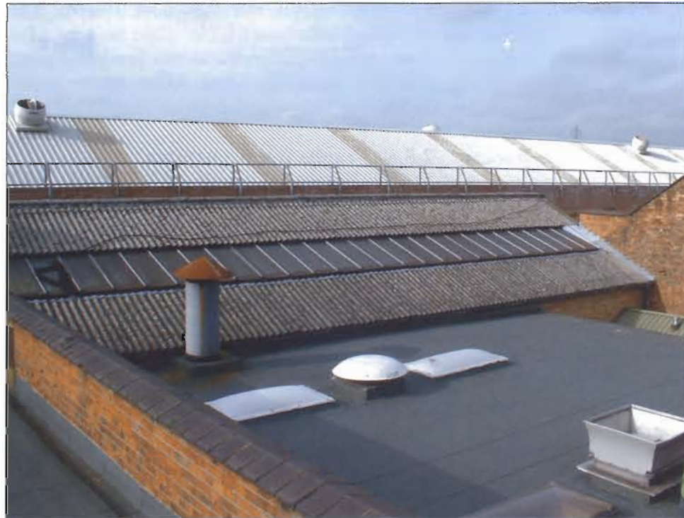
Figure 2.57 Complex roof area with examples of roof lights, fragile surfaces and barriers providing collective protection.
