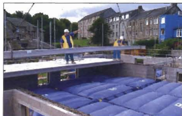
Figure 2.2 Air bags on construction site. (Photo: Health and Safety Executive)
