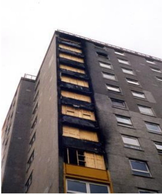
Figure 4: Post-fire damage illustrating the result of the Coandă effect
