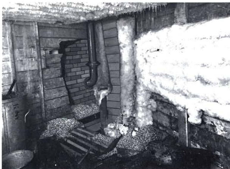
Plate 40. Results of a fire in an old type of cold store. The space between the brickwork and the wood panelling was filled with granulated cork. The fire spread from the compartment below up the chase left for the pipework. (Section 12).
