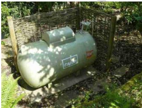
Figure 2: LPG storage tank – photograph courtesy of Peter Martin
