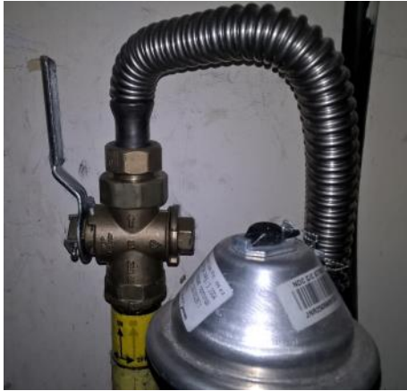
Figure 1: Gas isolation valve – photograph courtesy of Janet Guthrie
