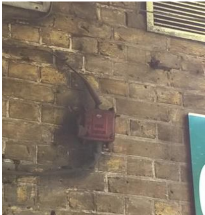
Figure 12: Fire switch for luminous discharge tube sign – photograph courtesy of Janet Guthrie
