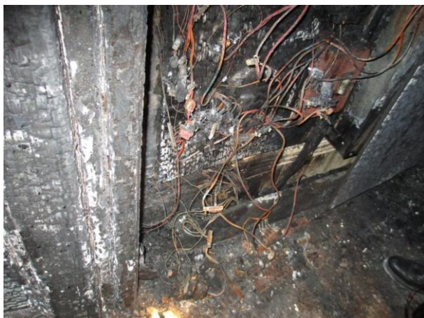
Figure 10: Damaged wiring due to a fire – photograph courtesy of Peter Martin
