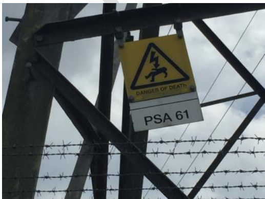
Figure 7: Identification number plate on transmission tower – photograph courtesy of Peter Martin
