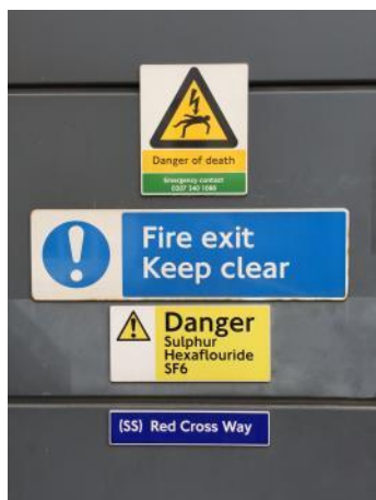
Figure 9: Substation access door (also showing SF6 warning sign) – photograph courtesy of Peter Martin
