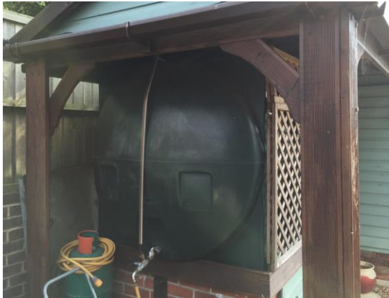
Figure 4: Fuel oil tank – photograph courtesy of Peter Martin
