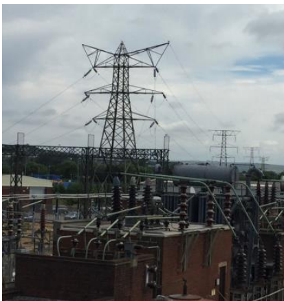
Figure 6: 132kV transmission towers – photograph courtesy of Peter Martin
